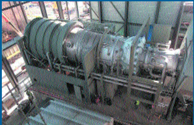
The gas turbine – the power engine of the new Coolkeeragh ESB power plant – installed on site
